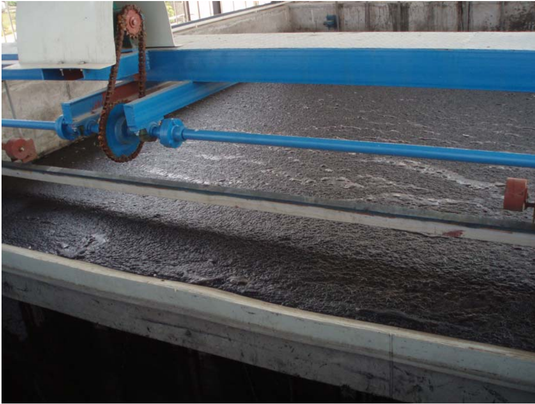
Photo 3: Concrete Dissolved air floatation with sludge scraper
