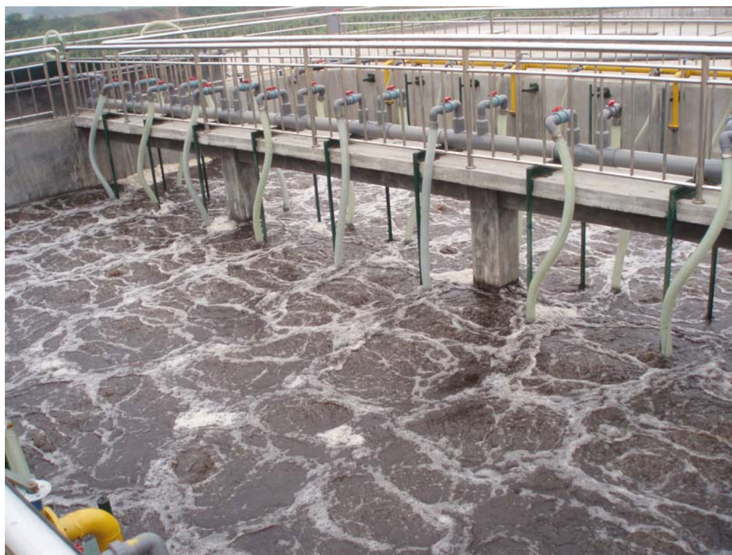
Photo 5: Membrane Bioreactor tank with submerged membranes
